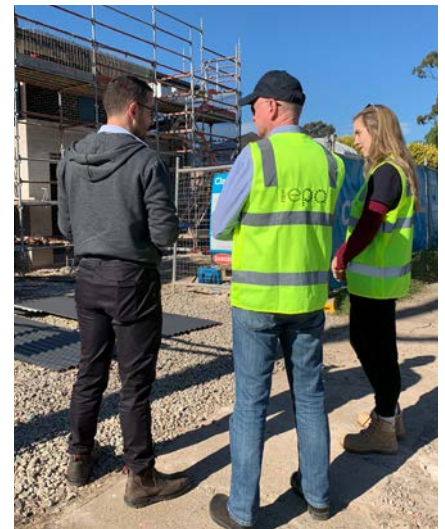
EPA staff alongside local council examine a construction site in Blacktown as part of the Get the Site Right Blitz Day. Photo: EPA
