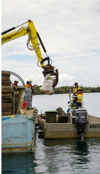
Heavy machinery is used in the clean-up effort along the Tweed River. Photo: EPA
