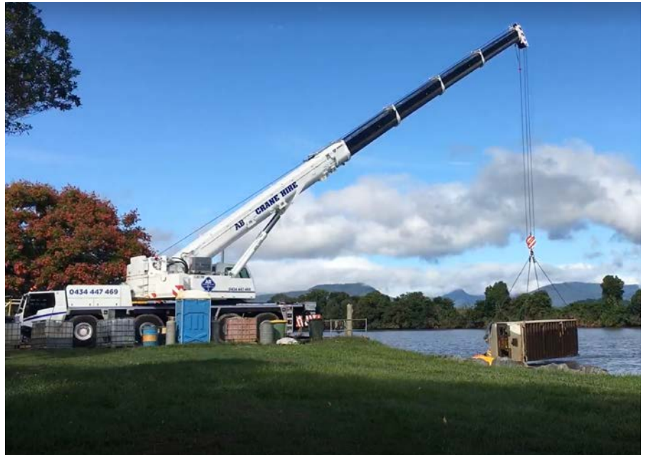
The crane lifting a waterlogged Ernie out of the river. Photo: Nicholas Payne/EPA
