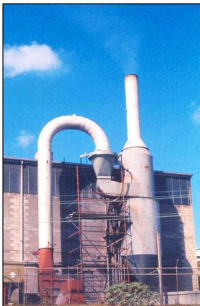
Venturi scrubber for metallic fume
