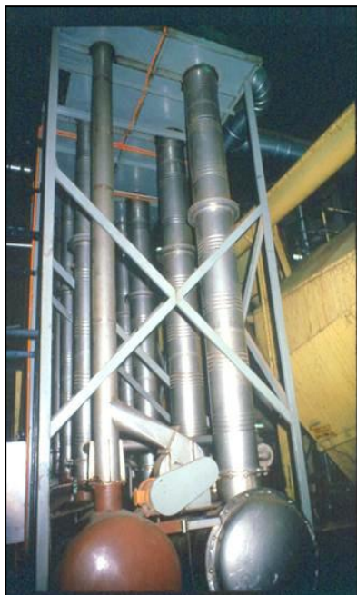
Shell and tube condensers for wet rendering gases before incineration
