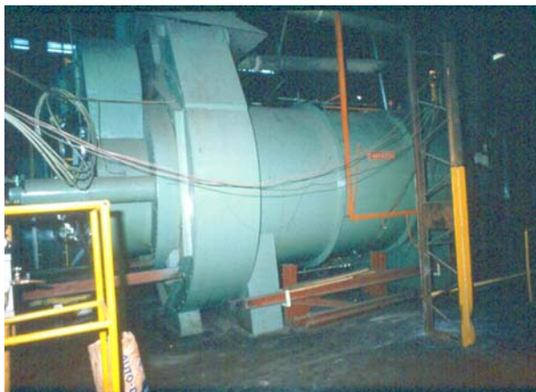
Fume incinerator for building materials
