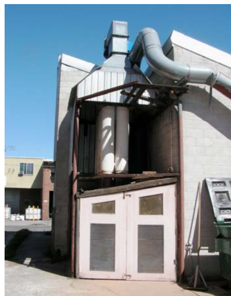
Small baghouse collecting saw dust from a suburban joinery shop
