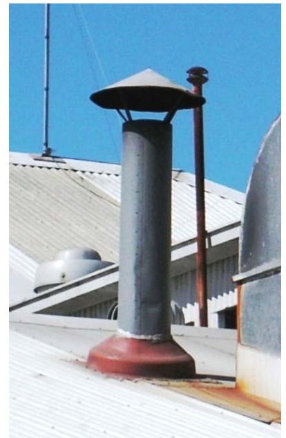
This sort of stack cover should be avoided as it reduces the plume rise.
