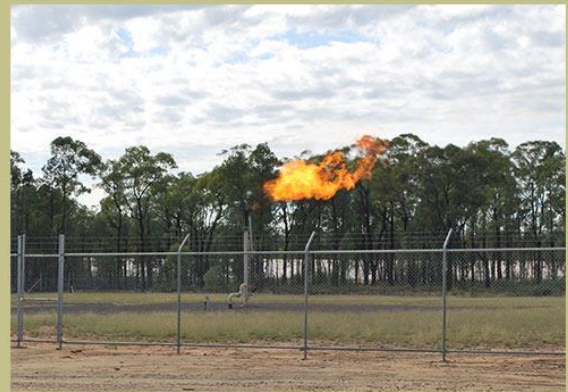
Example of an open vertical flare at a NSW coal seam gas site.
