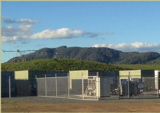
Example of an enclosed flare at a NSW coal seam gas site.
