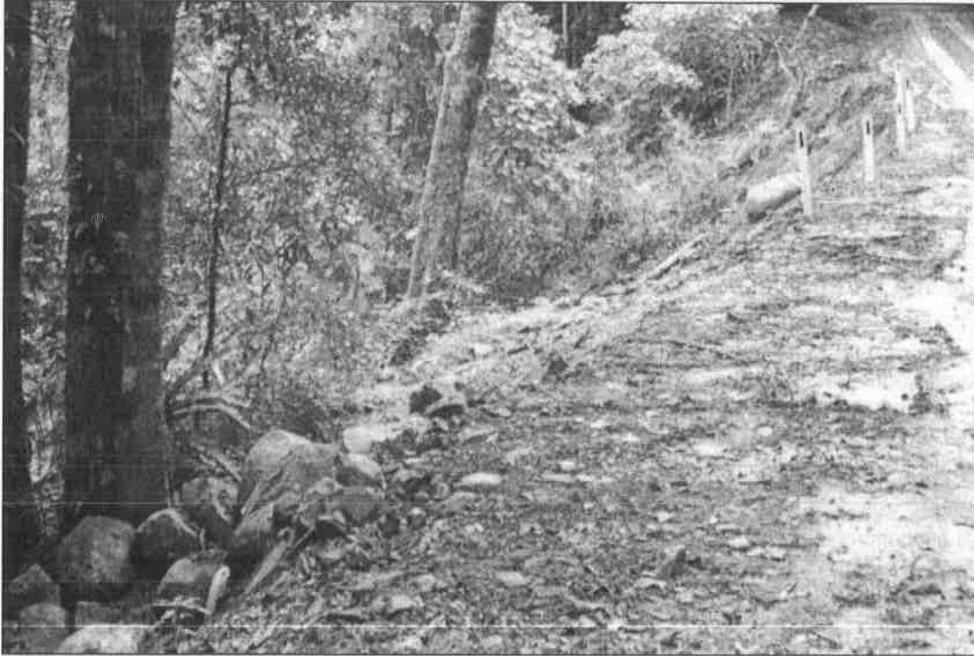
Figure 5. Sheet erosion and roadside slumping.
