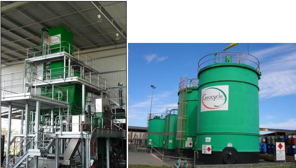
Figure 29: Geocycle de-packaging unit and blended fuel storage tanks
