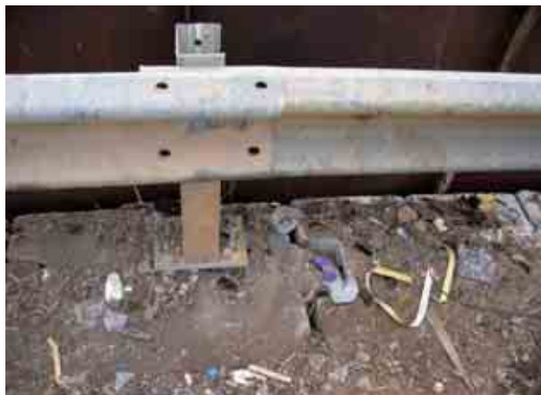
Photo 33.2 Platform movement due to ground settlement
