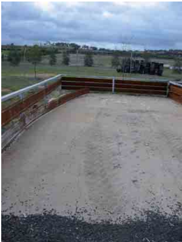
Photo 27.11 Damage to storage bay
