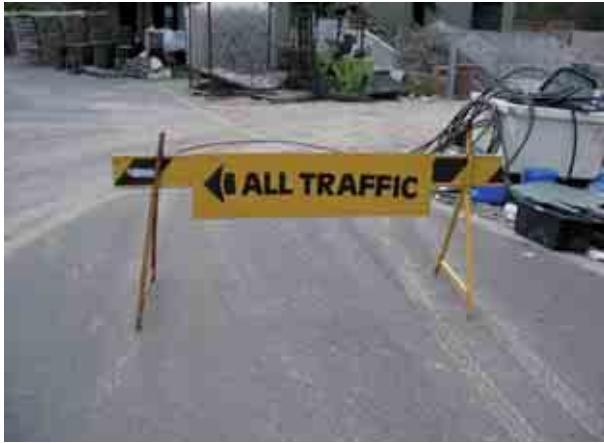
Photo 35.1 Signage to direct traffic flow
