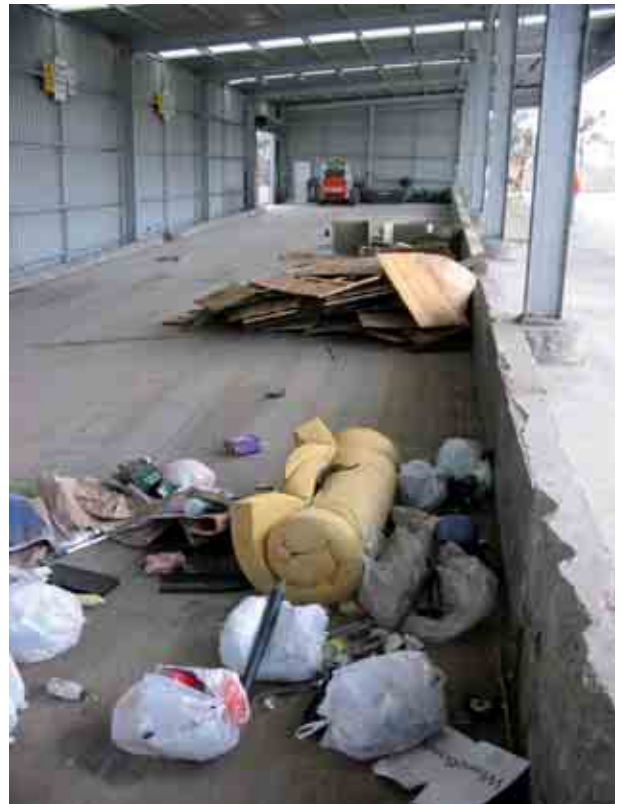
Photo 36.8 Waste disposal area with damage to retaining wall
