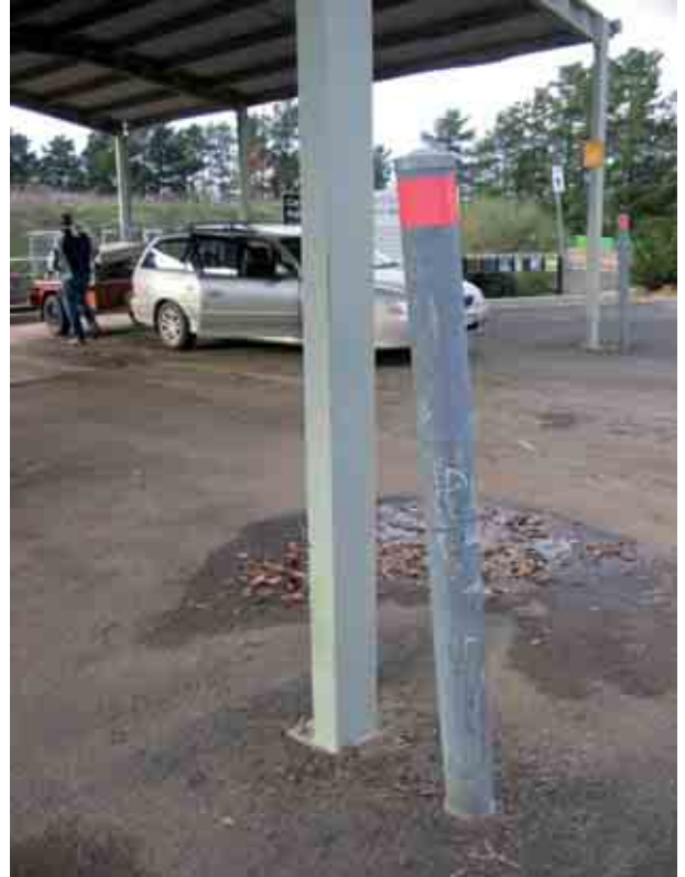
Photo 28.13 Bollard protecting vertical support beam
