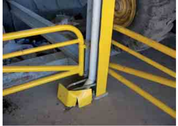
Photo 30.21 Controls in place to minimise damage from vehicles
