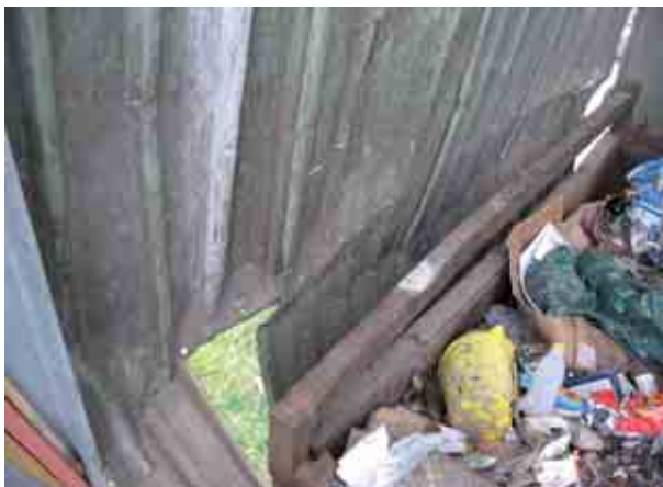
Photo 35.6 Damage to shelter
