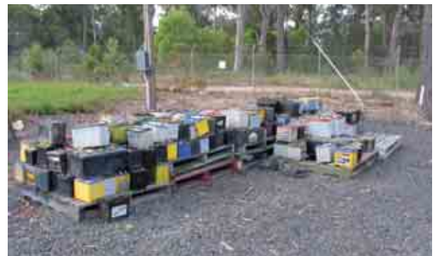
Photo 37.8 Stockpiled lead acid batteries (Note: Batteries should be stored in a covered and bunded area)
