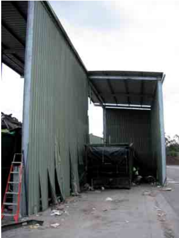
Photo 35.4 Damage to shelters from transfer bins and trailers
