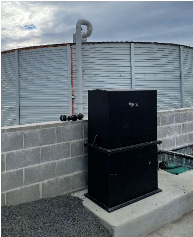
Figure 13 Activated carbon filter for leachate
