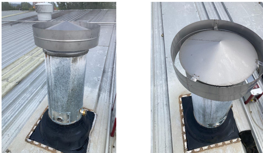
Figure 2 Example of a rain cap over the outlet of a stack, which should be avoided since it inhibits dispersion
