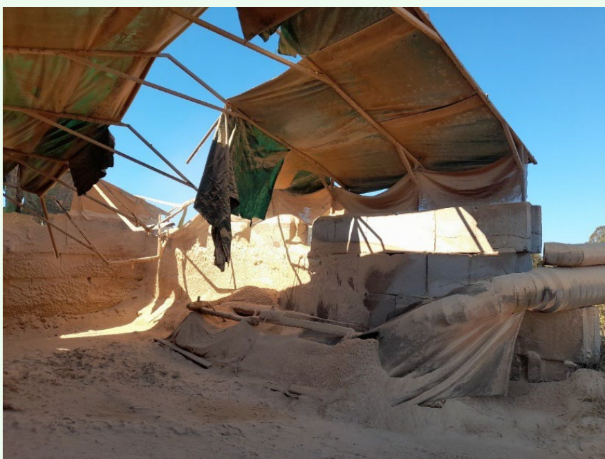
Figure 5 Inadequate construction and maintenance resulting in failure of a dust storage facility at a wood processing premise
