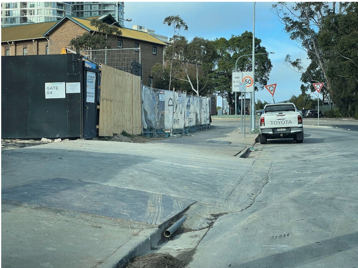
Figure 1 Tracked out material that has dried on the road surface becomes a dust source Source: Jane Barnett/Zephyr Environmental
