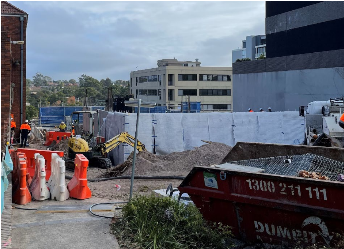
Figure 6 Example of additional or temporary sheltering erected within a construction site for higher dust generating operations Source: Jane Barnett/Zephyr Environmental
