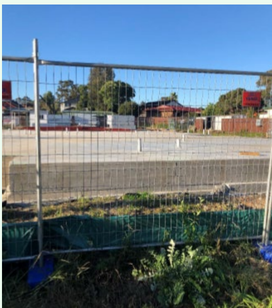
Figure 8 A fence without dust screens
