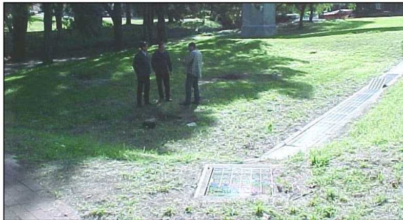
Figure 3.2. Infiltration basin located in Annandale used for detaining stormwater run-off from surrounding streets and filtering prior to discharge to Whites Creek and Sydney Harbour.
