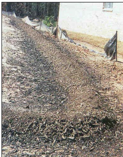
Figure 4.3. A compost filter berm replaces a failed silt fence, shown in the background (Goldstein, 2001).
