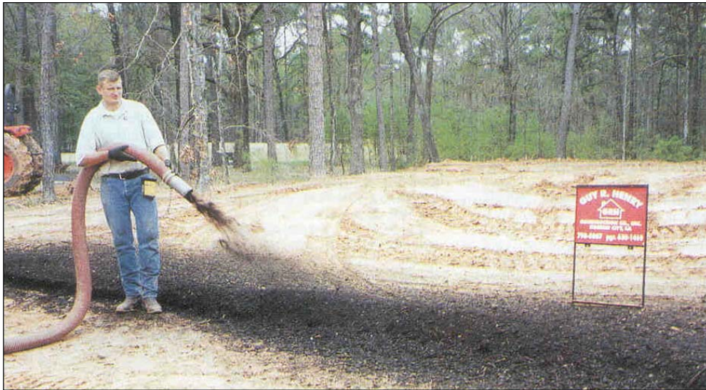
Figure 4.4. A filter berm used around a construction site to trap sediment. This berm is constructed from a 50:50 mix of compost and mulch and applied using a pneumatic blower (Goldstein, 2001).
