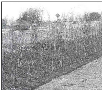
Figure 4.1. Compost berms at the base of slopes are effective for erosion and sediment control (Alexander, 1999).
