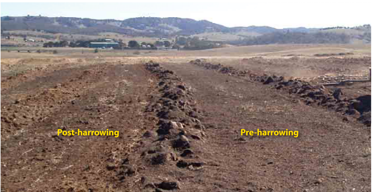
Figure 9. Harrowing is done to incorporate the soil conditioner and seed into the topsoil to protect it from drying out and blowing away. This also aids in vegetation establishment.
