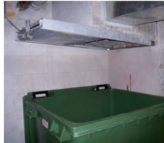
Garbage chute emptying into skip
