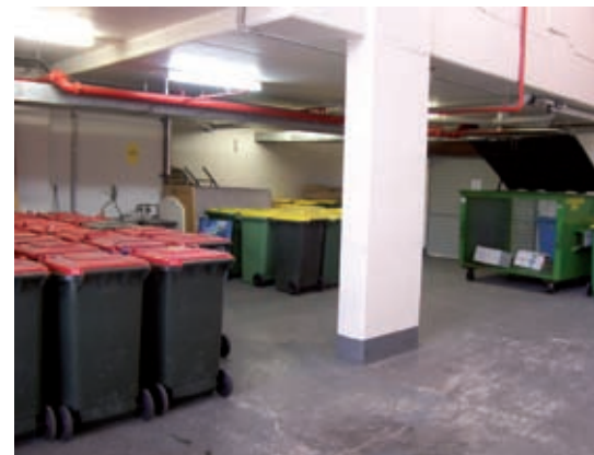
Segregation of garbage and recycling in the residential central storage and collection area
