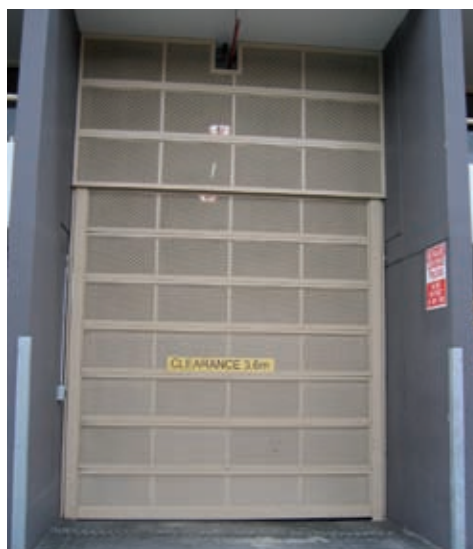
Expanded metal door entrance to the central storage and collection room from street level
