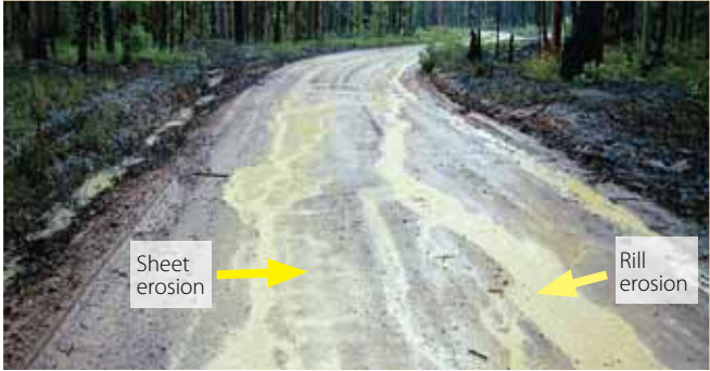
(a) Rill and Sheet erosion
