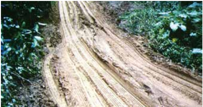
Figure 5.27: Example of road surface breakdown
