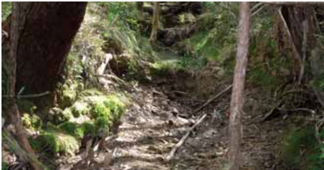
(b) Gully erosion
