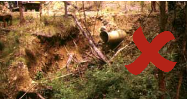
Figure 5.16: Example of poor outlet protection
