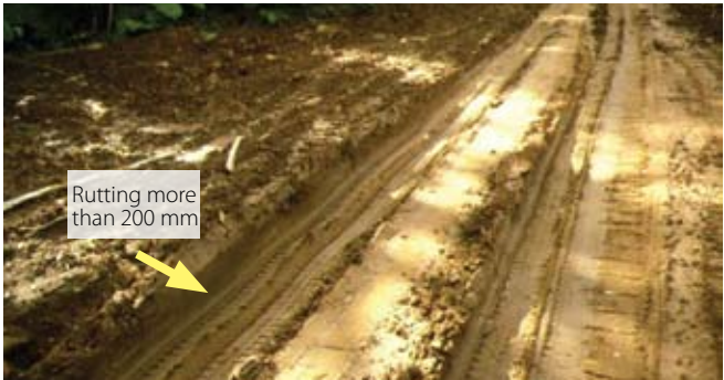
Figure 5.27: Consequences of using roads in wet weather
