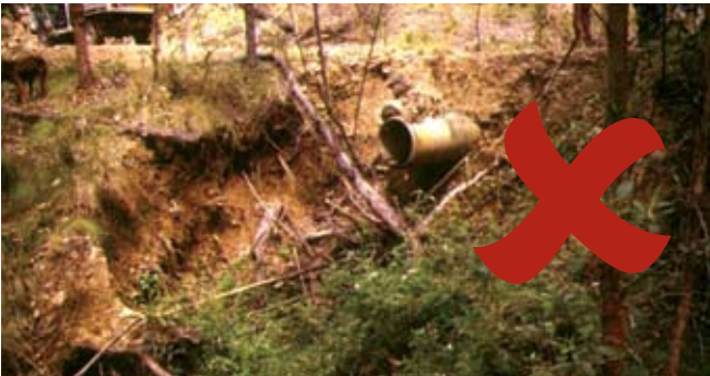
Figure 5.16: Example of poor outlet protection
