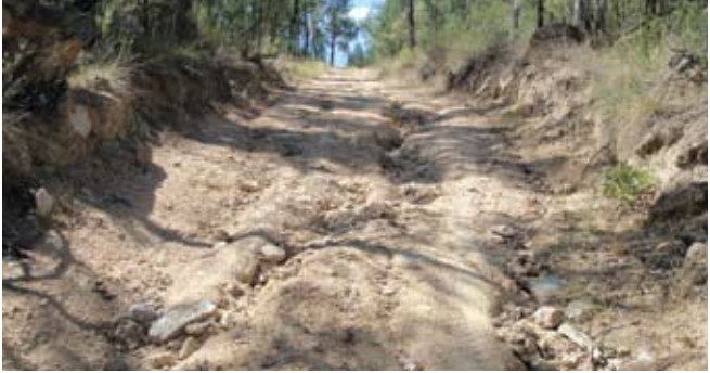
Figure 5.28: Example of road surface breakdown
