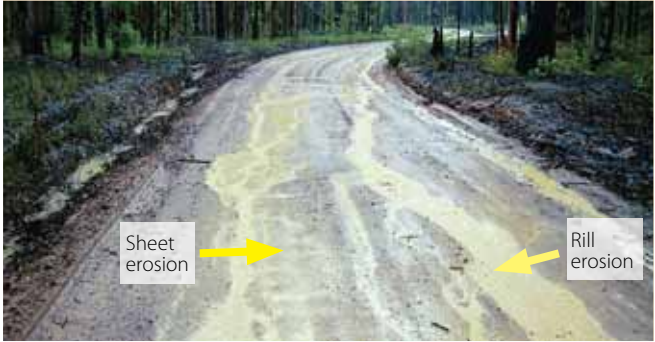
(a) Rill and sheet erosion
