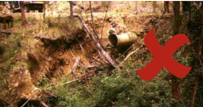
Figure 5.16: Example of poor outlet protection
