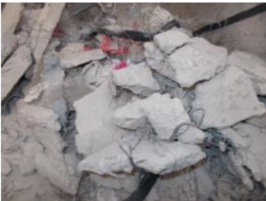
Broken concrete pieces
