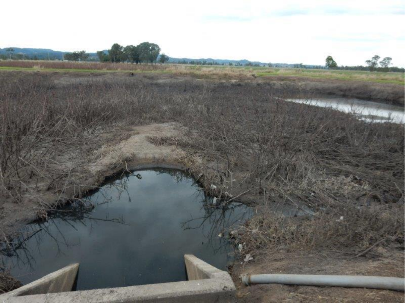
Photo 14: Emergency storage pond used for trade waste, posing a risk of stormwater and groundwater pollution
