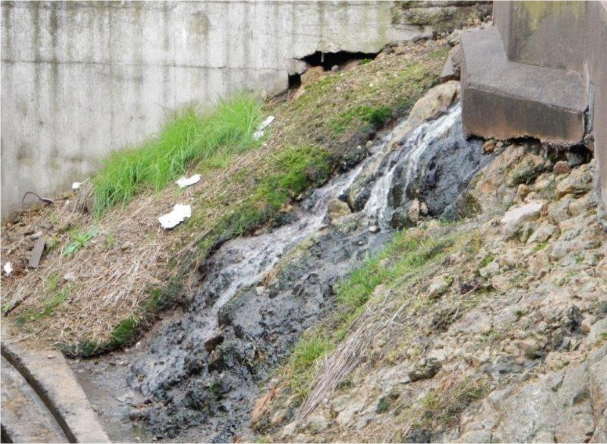
Photo 17: Wastewater discharging from a leak in a concrete channel (lack of maintenance)
