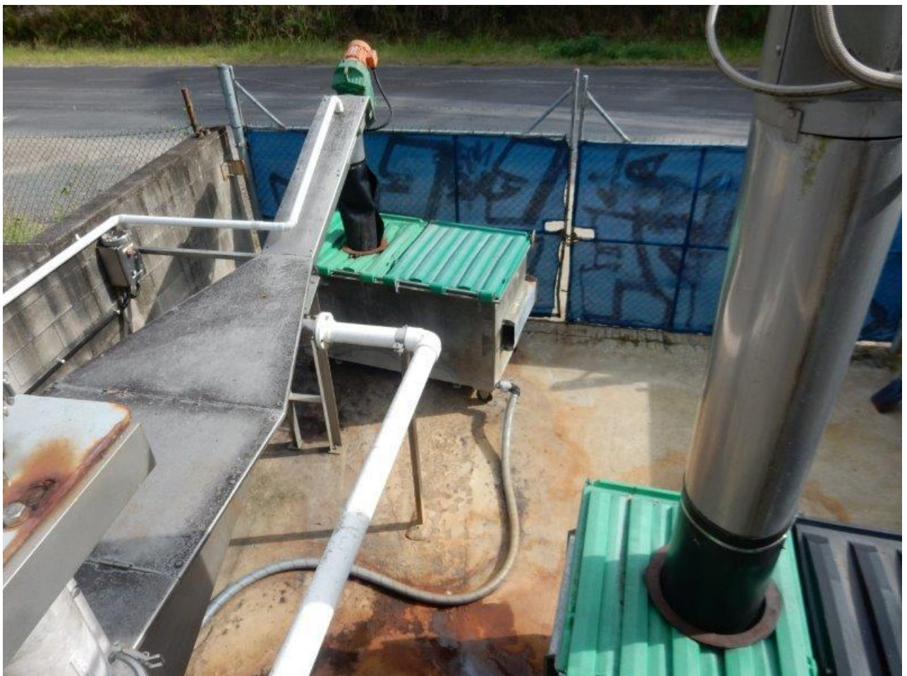
Photo 2: Enclosed grit collection
