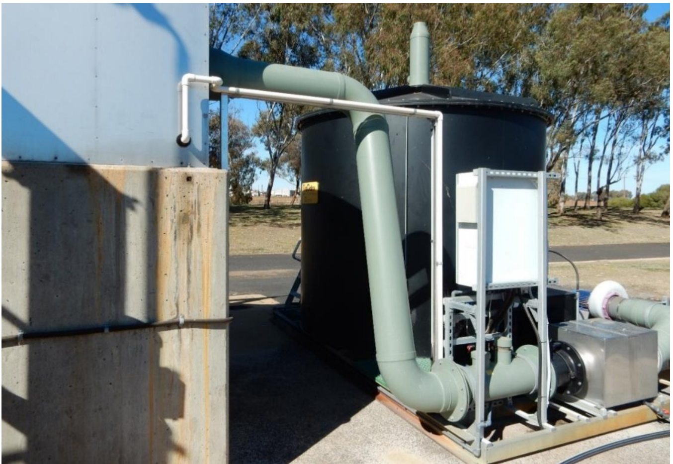
Photo 20: Enclosed inlet works with odour control unit
