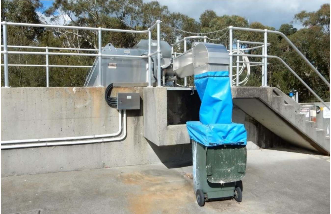
Photo 21: Inlet works with covered screening bin
