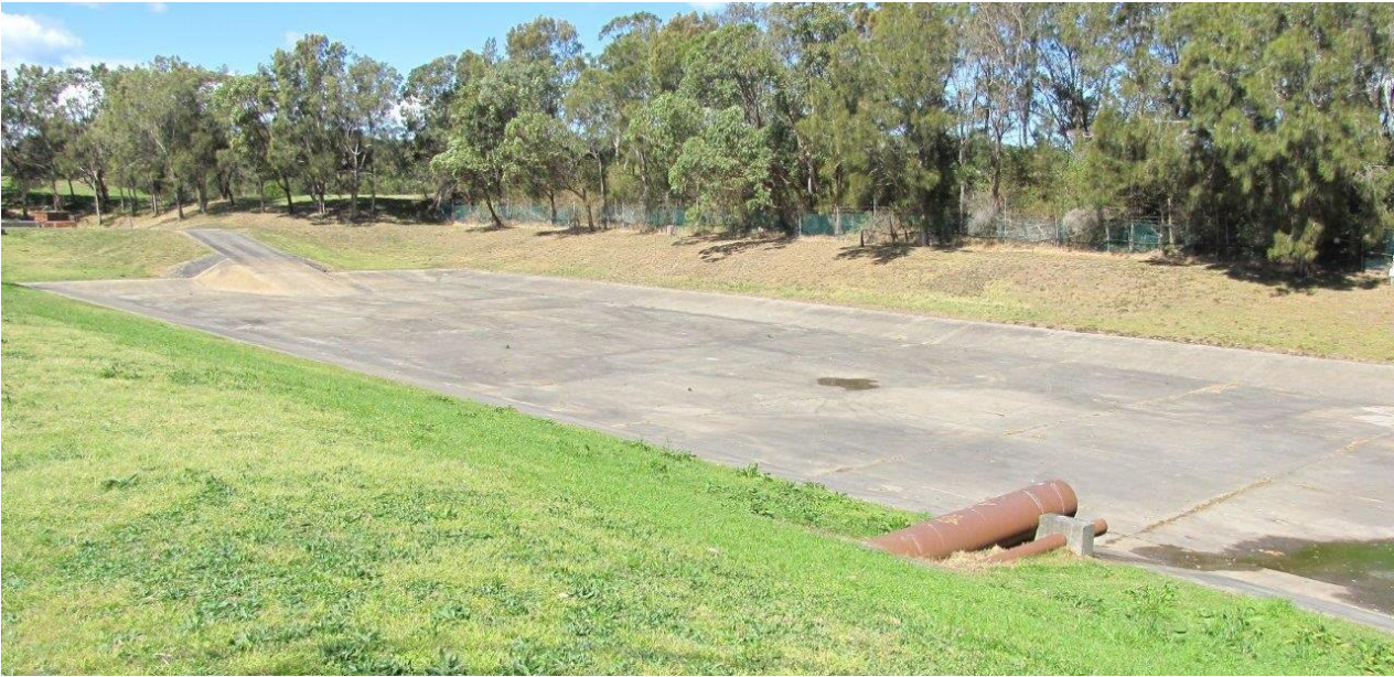
Photo 19: Emergency storage pond
