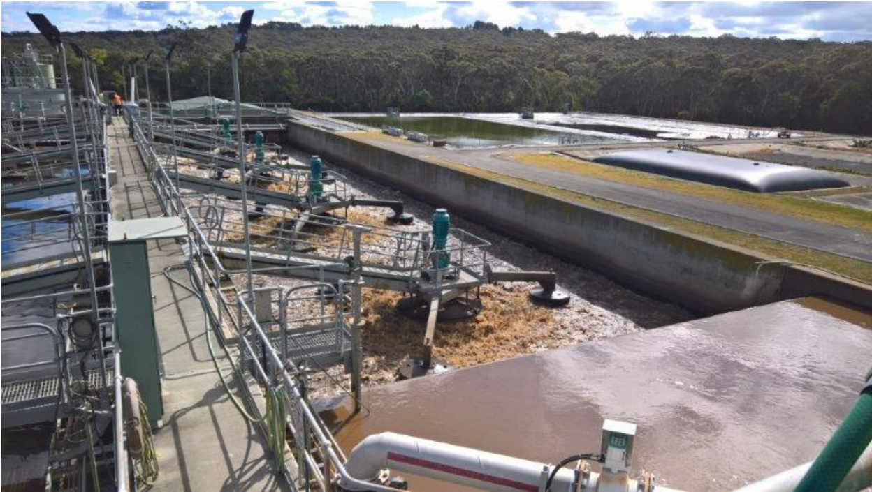
Photo 9: IDEA tank in aeration with sludge lagoons and sludge drying bag in background
