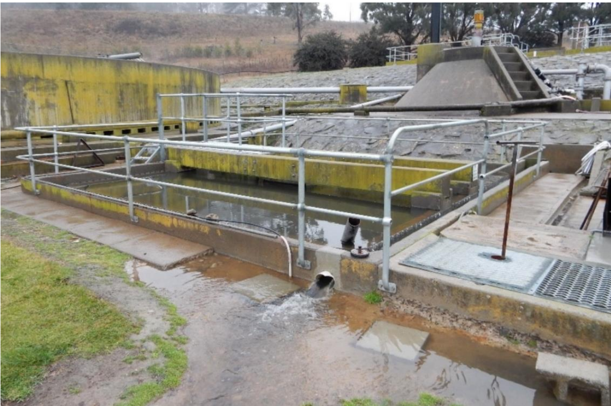
Photo 18: Effluent pooling around temporary discharge point, presenting a risk of land and water pollution
