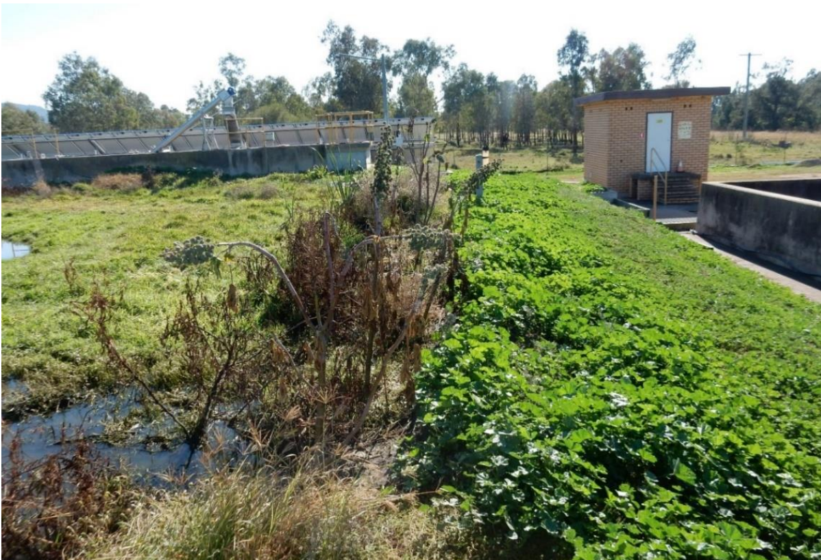
Photo 15: Active sludge lagoon with grass growth, indicating inadequate sludge management and lack of maintenance
