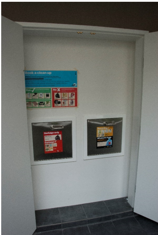
Example of a dual waste and recycling chute inlet in a bin cupboard in a low-rise residential building (Photo: Andrew Quinn)
