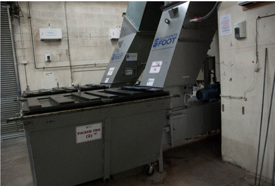
Two x 3 m3 bulk bins attached to a small-scale static compactor at the base of a chute (Photo: Andrew Quinn)
