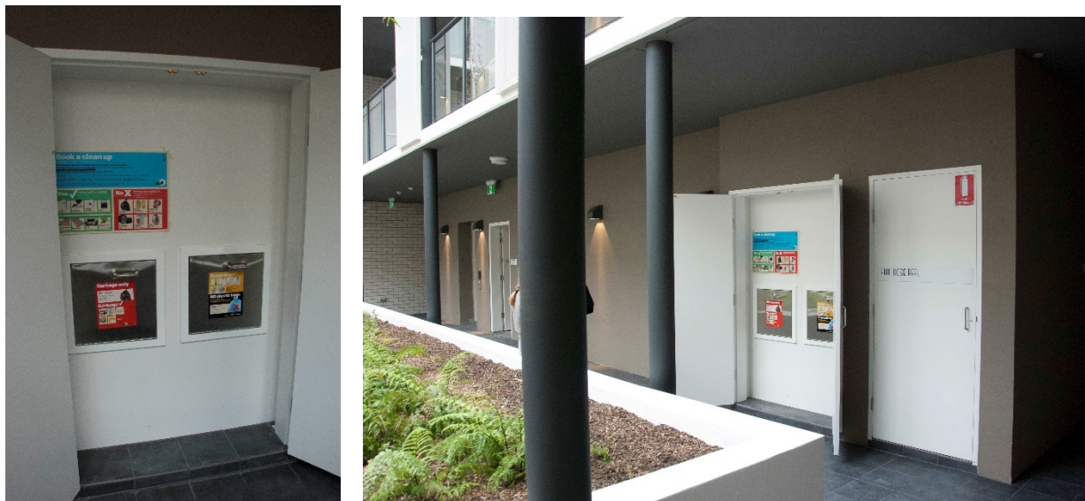
Bin cabinet containing the dual waste and recycling chute hoppers (Photo: Andrew Quinn)
