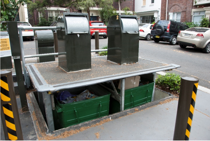
Example of an underground bin system in Sydney used by the residents living in residential flat buildings in the surrounding area (Photo: Andrew Quinn)
