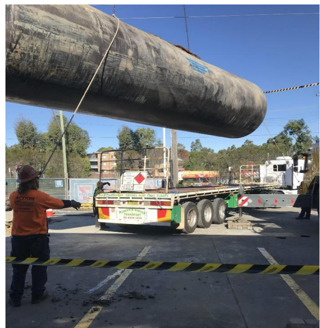
A tank is removed from the ground and transported for appropriate disposal as part of the decommissioning process.
