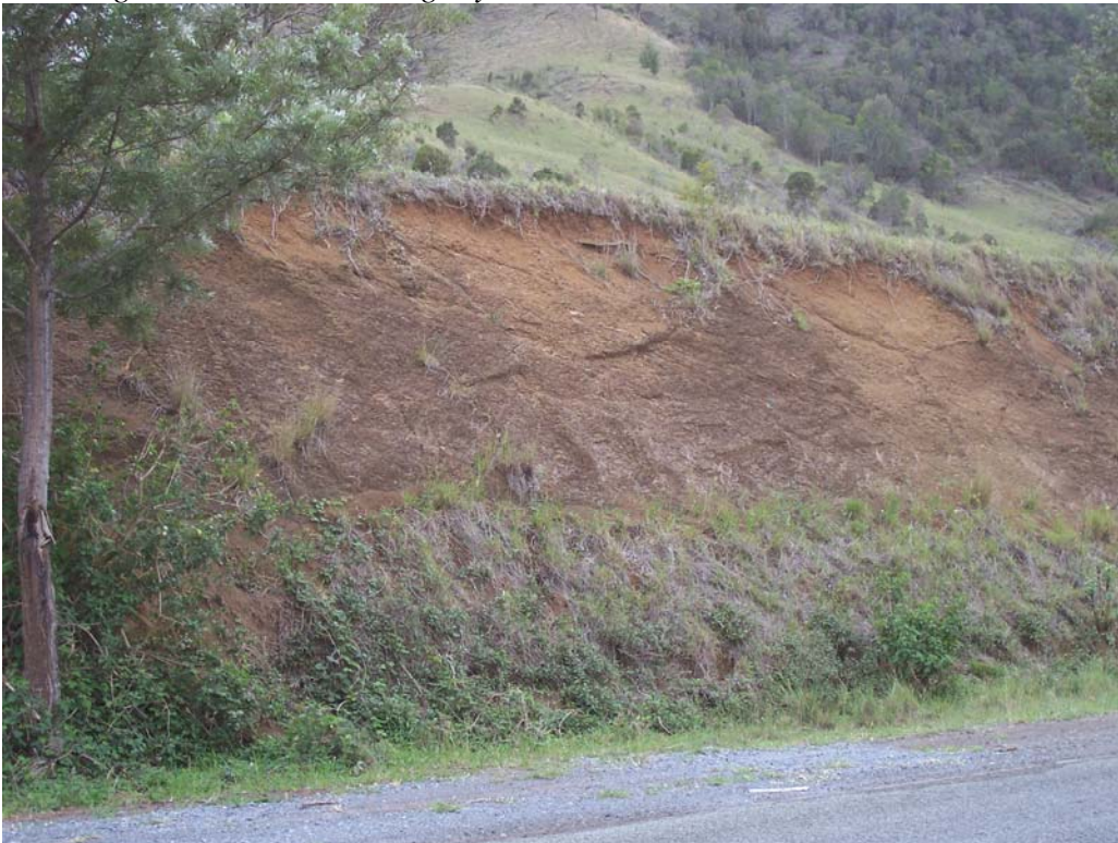
Photo 4 Deep fertile permeable non cracking clay soils on basalt – prone to land slips terracing and sheet erosion – gully and tunnel erosion rare
