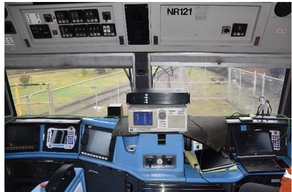
Power measurement device installed in cabin
