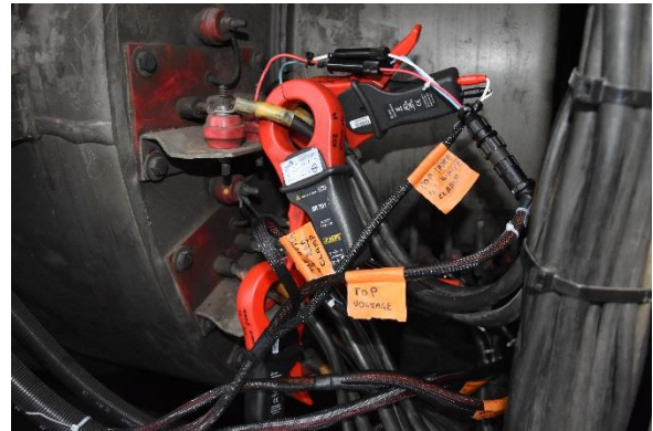
Current clamps for battery & auxiliary alternator
