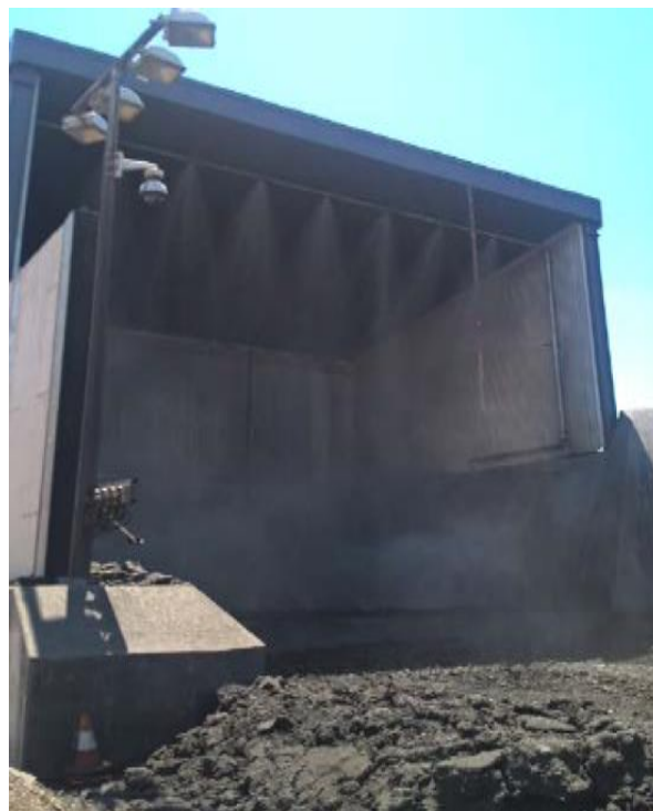
Figure 23 ROM bin at MCCM with water sprays in operation
