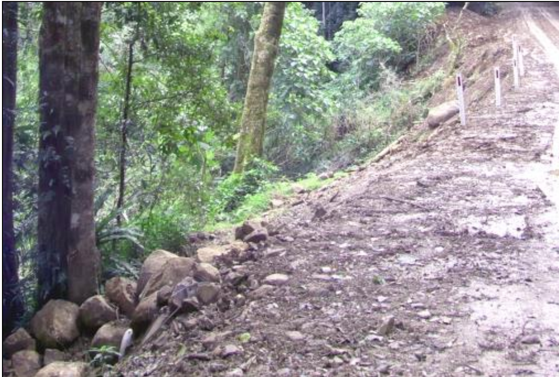
Figure 5. Sheet erosion and roadside slumping.
