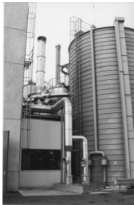
Figure 5-3 Residual waste gasification
