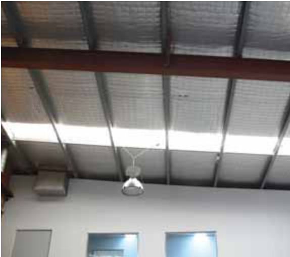
Significant energy savings can be achieved by installing skylights and roof insulation and by using energy efficient lighting.
