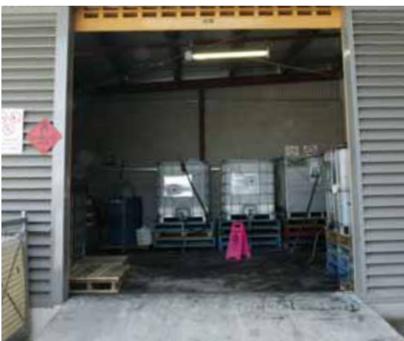
Store drums of chemical waste awaiting collection in a covered and banded area. Ensure there is no possibility that waste chemicals could be washed into gutters or drains, or into the sewer.
