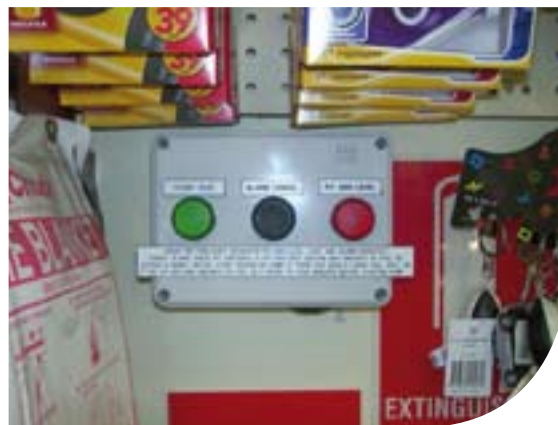
A collection pit alarm can prevent contaminated water finding its way into the stormwater system.
