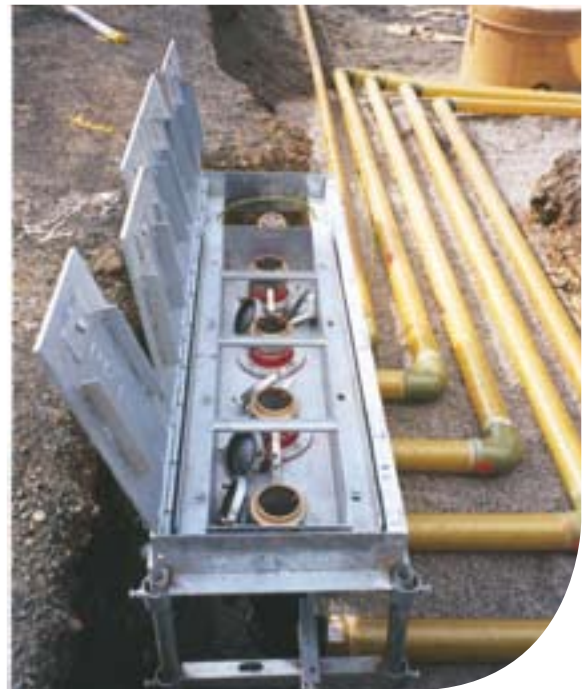
Typical remote fillbox incorporating spill containment to prevent accidental releases entering the environment.
