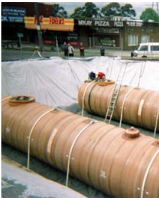
Double walled tank installation with excavation lined with geo-fabric to prevent migration of native soil into the backfill material.
