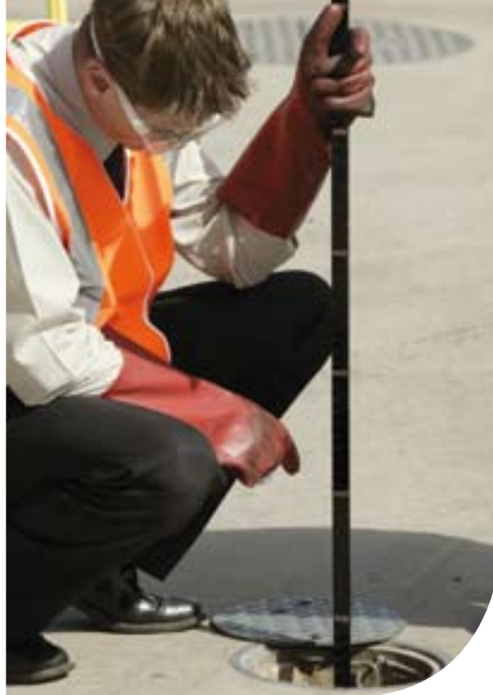
Ensure underground fuel tanks are checked regularly for fuel leaks and water infiltration.
